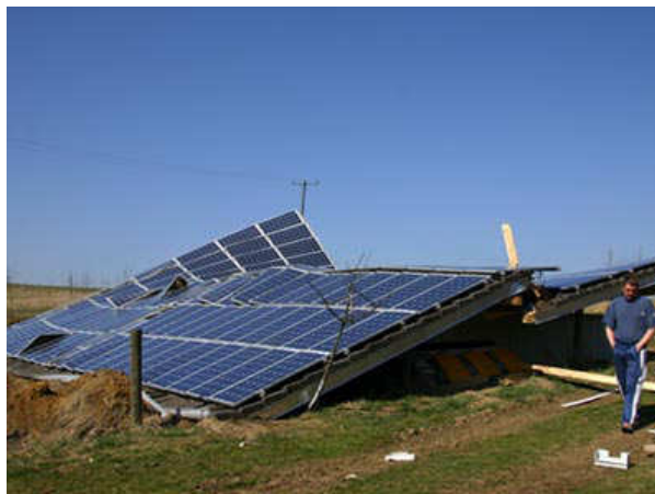
Image 5: Storm damaged modules
