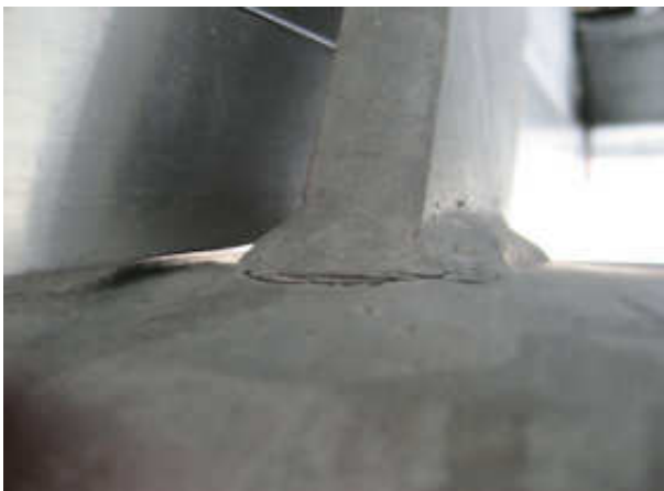
Image 4: Crack damage – fixing system
