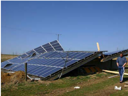
Storm damaged modules
