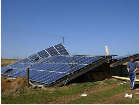
Storm damaged modules
