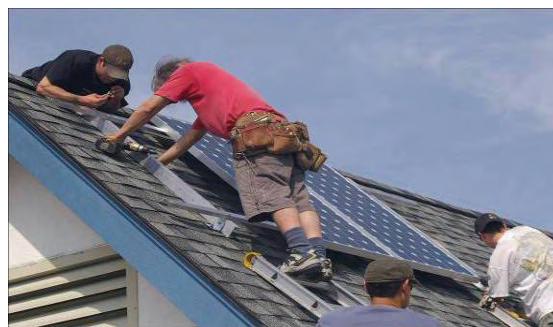
Figure 7: PV installation on building
